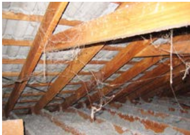
Loose-fill asbestos is considered the world's most dangerous asbestos product. (Supplied: WorkCover NSW)
