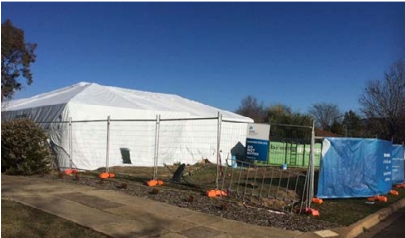
Felicity Prideaux says a dome was placed over her house so that it could be demolished safely. (Supplied: Felicity Prideaux)
