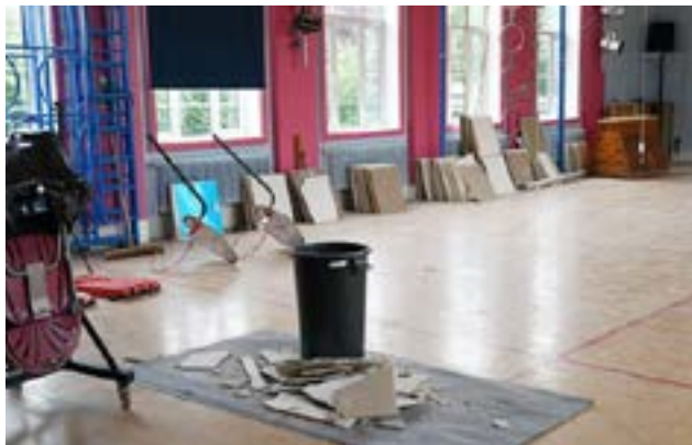
This primary school in Leicester is among the dozens that have affected by unsafe concrete. Jacob King/PA images
