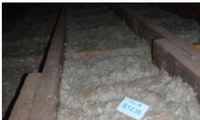
Loose-fill insulation in a roof space. (Supplied: Robson Environmental)
